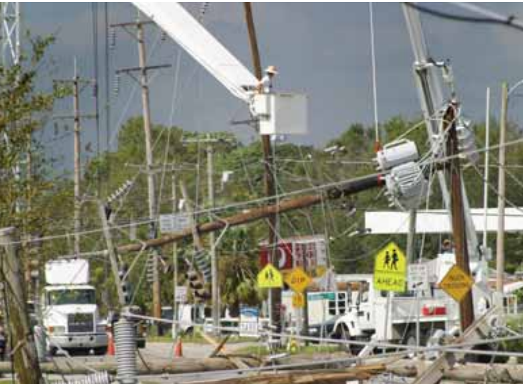
Devastation in Auburndale, Fla. shows the amount of damage endured by Tampa Electric's system during the 2004 hurricane season.
