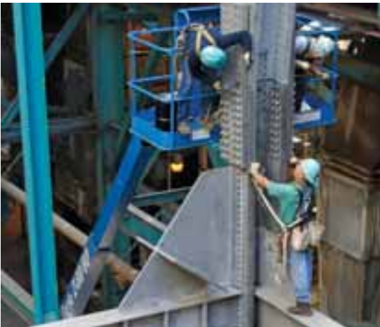
Tampa Electric team members install pollution control equipment at Big Bend Power Station.
