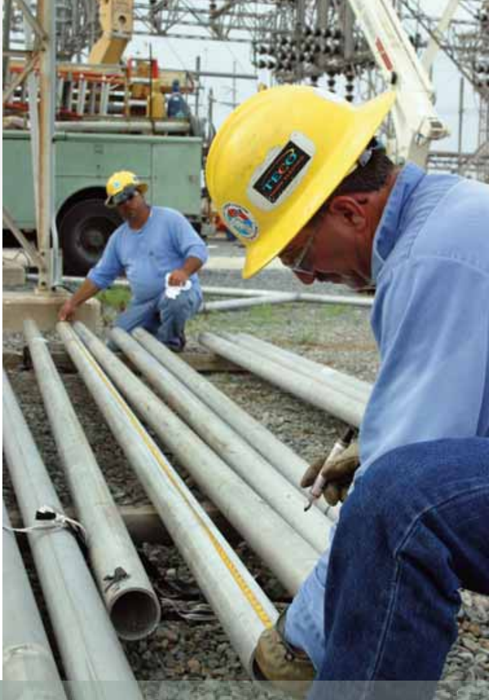
Team members at work in the switchyard at Tampa Electric's H.L. Culbreath Bayside Power Station.
